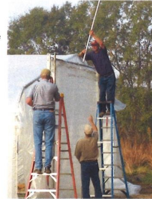
Volunteers place the final plastic panels on the high tunnel garden to complete the structure.
